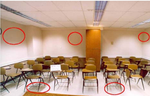
Figure 6: Open-cell Parabolic Fixtures
